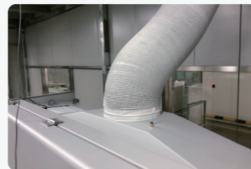
Exhaust Hood and Pipe
